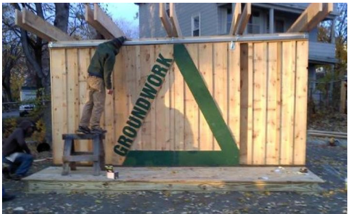
Green Team, GWL staff, and Farm School building a tool shed and hoop house at Giuffrida Community Garden
